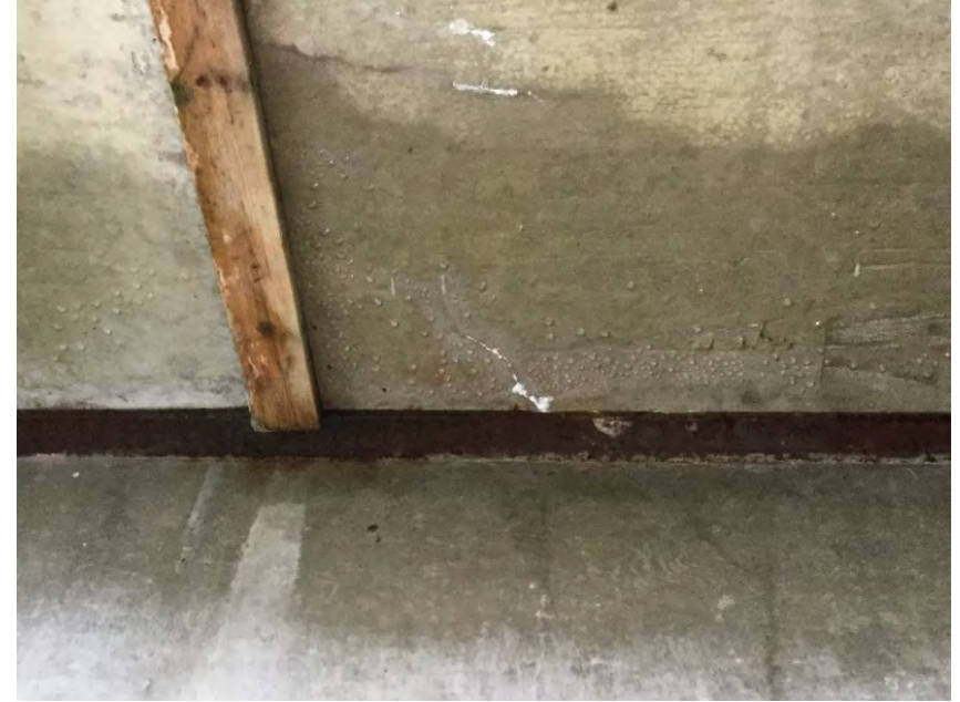
Minor cracking and efflorescence noted on panel 1 right bank
