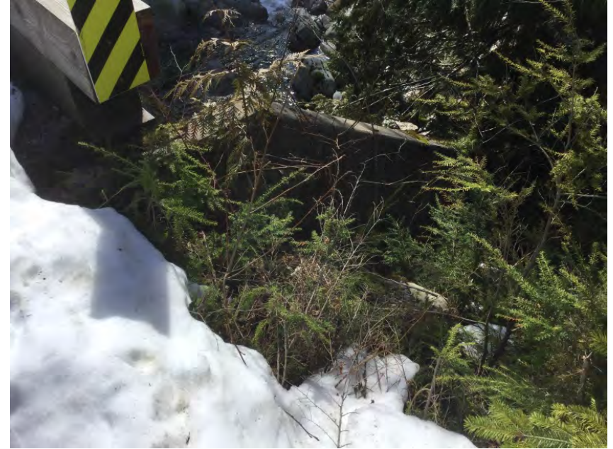
Fill eroding at downstream right bank
