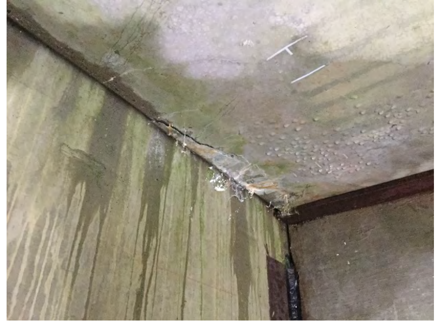
Minor damage noted to panel 1 at left bank
