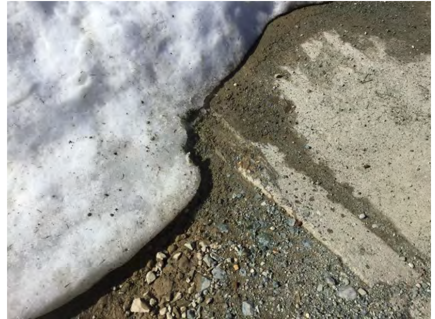
Minor damage noted to top of ballast wall at left bank
