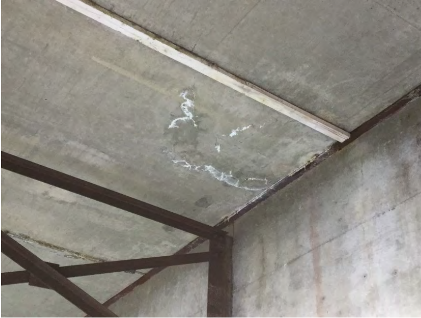
Minor cracking and efflorescence on Center panel
