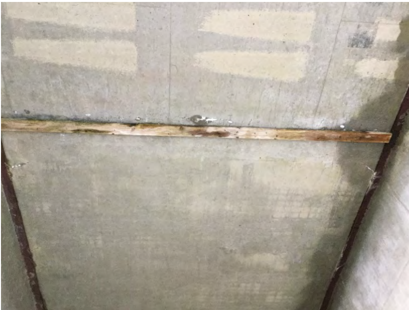
Minor cracking and efflorescence on panel 1 and 2 at left bank
