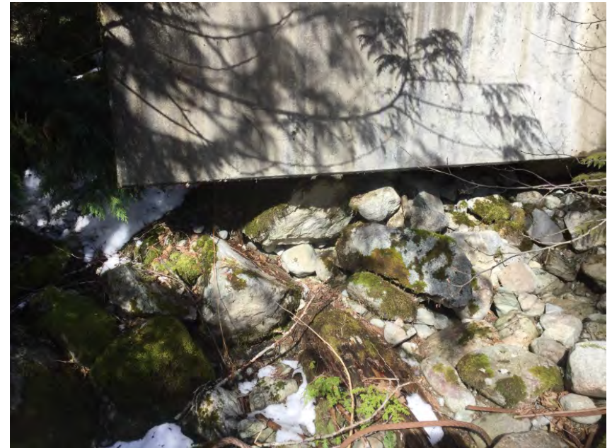
Fill eroding at downstream right bank
